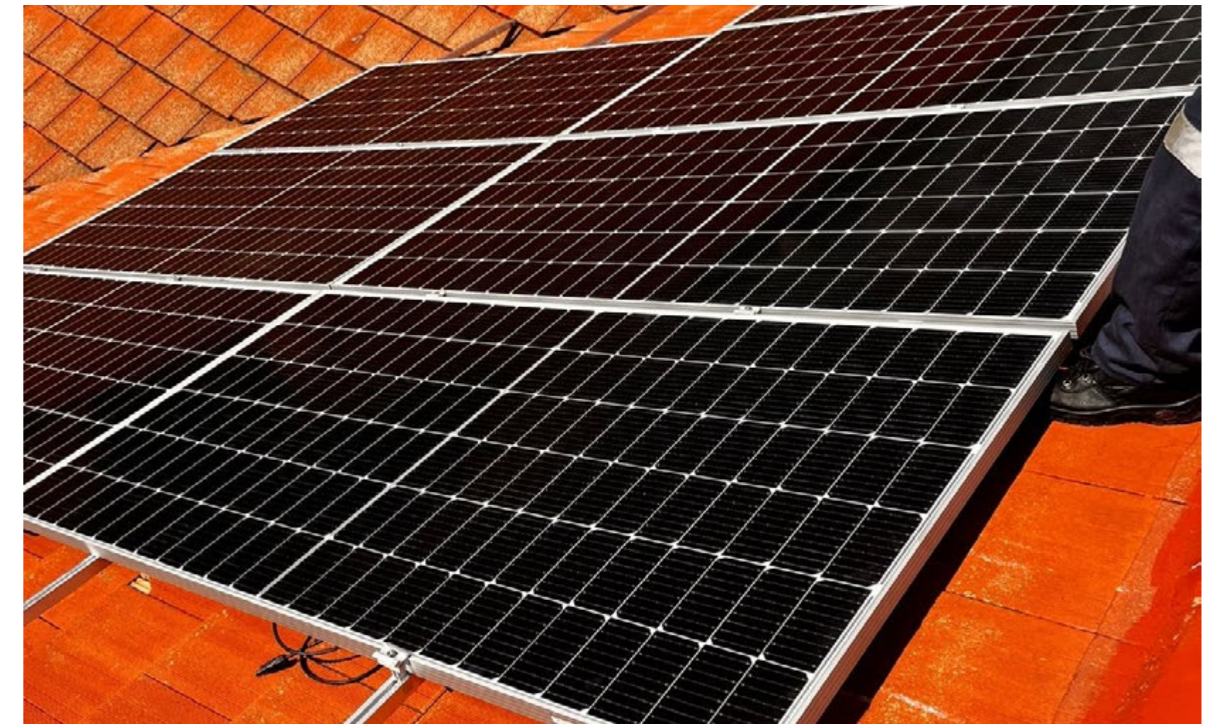
Nedlac has installed a new solar inverter at their offices in Johannesburg.
